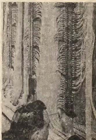
This is part of a mammoth wiring job which has recently been carried out at Tyne Tees Television's enlarged and re-equipped City Road Centre in Newcastle. The photograph shows vision wiring on the termination panel of the central camera control, for which British Insulated Callender's Cables Ltd. supplied over 40 miles of cable.
